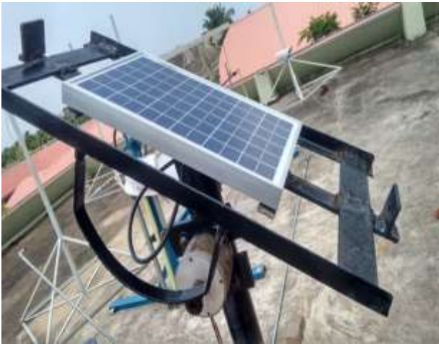
Fig. 2. Solar PV tracker setup installed by the authors at their university.
