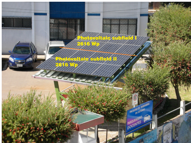
Figure 3. Distribution of photovoltaic subfields I and II on the metal support structure of solar Electric Vehicle Chargers.
