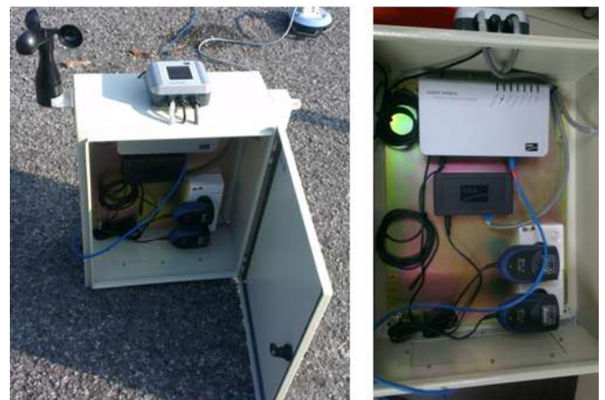
Fig. 5. Portable solar measurement system and data logger.
