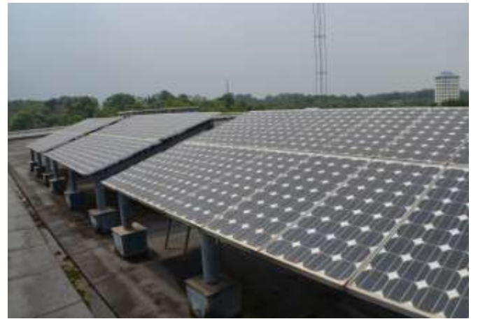
Fig. 7. The 3.15 kWp solar PV rooftop system.
