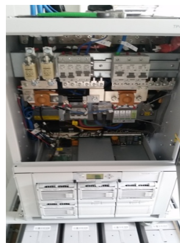
Fig.21. Lead Acid Battery bank system with the charge protection circuit
