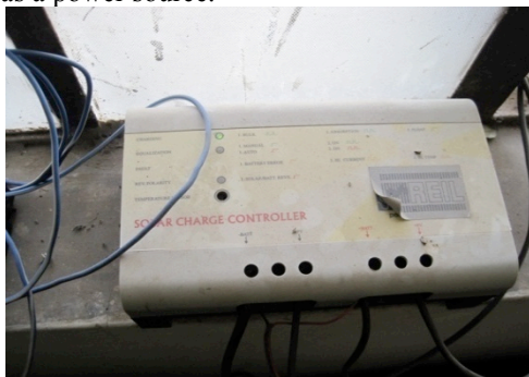
Fig.7. Solar charge controller
