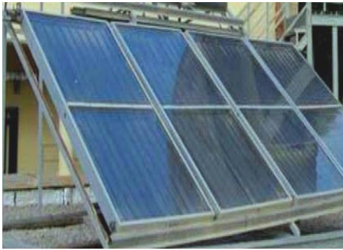
Fig. 2. View of the collector's field.
