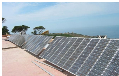
Fig. 9. PV panels in the roof of CDER.
