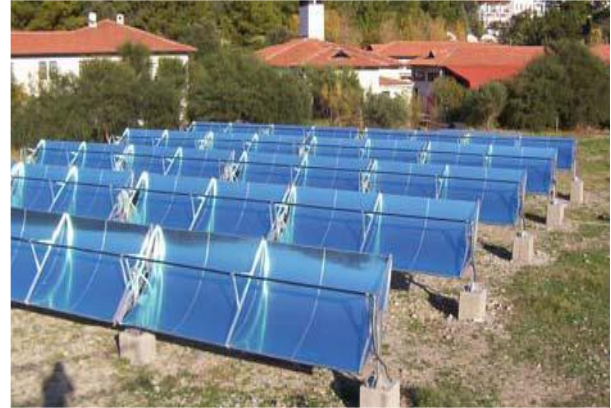
Fig. 6. Parabolic trough solar thermal technology [11]
