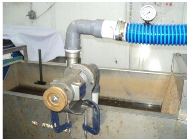
Fig 6. PAT is installed near the pressure gauge
