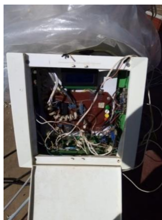
Fig. 29. The solar tracker control board.
