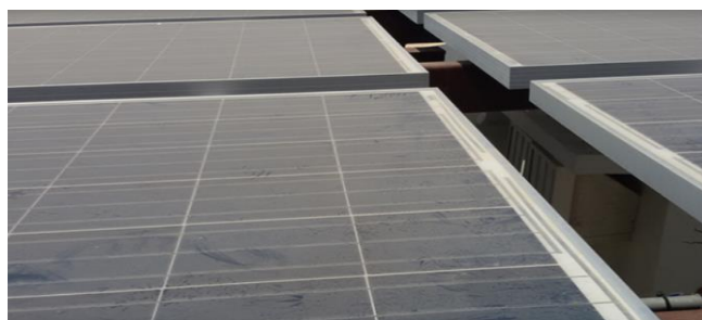
Fig.17. The dust on the surface of the solar panels
