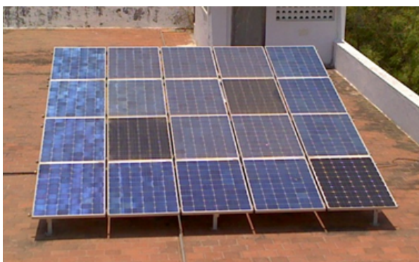
Fig. 14. Normal image of the 5kWp PV system
